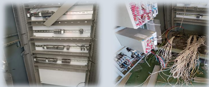
Photo 1: Vandalised MacDougall Street mini-substation
